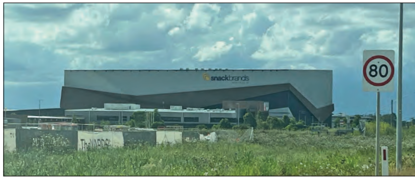
The new 30,255sq m Snack Brands Australia manufacturing and distribution facility under construction.
