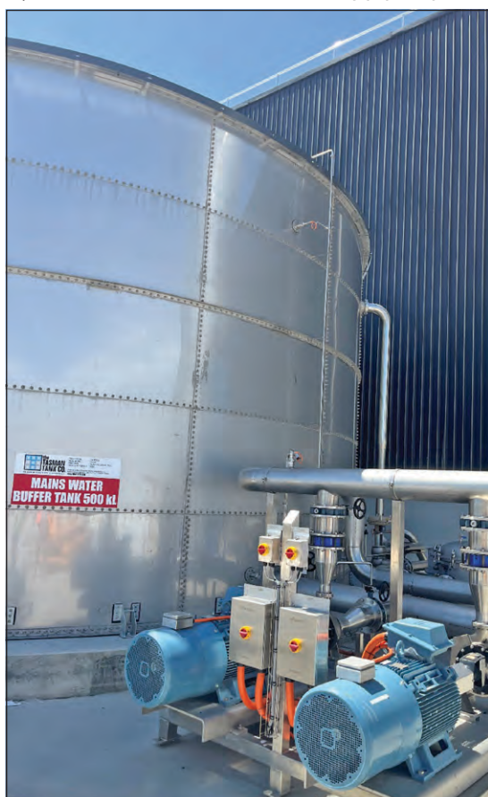
The on-site 500kL mains water buffer tank.
