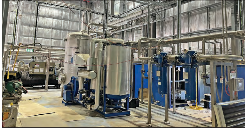
Three 110kW oil-free air compressors.
