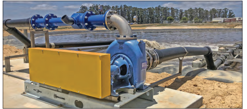
The EchoStorm 80 Series pump in situ, one of the best decisions Fletcher International Exports has made.
